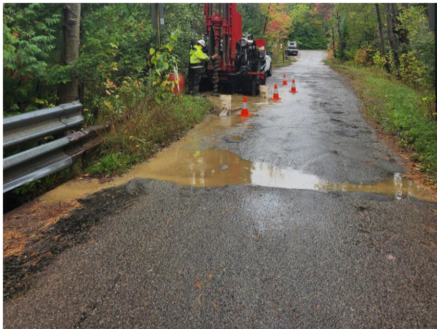
Photograph #2: View of Underhill Road from the existing north crossing. (Project No. 2023.1755, Underhill Road over Rapid River, Clearwater Township, Kalkaska County, Michigan, October, 2023)
